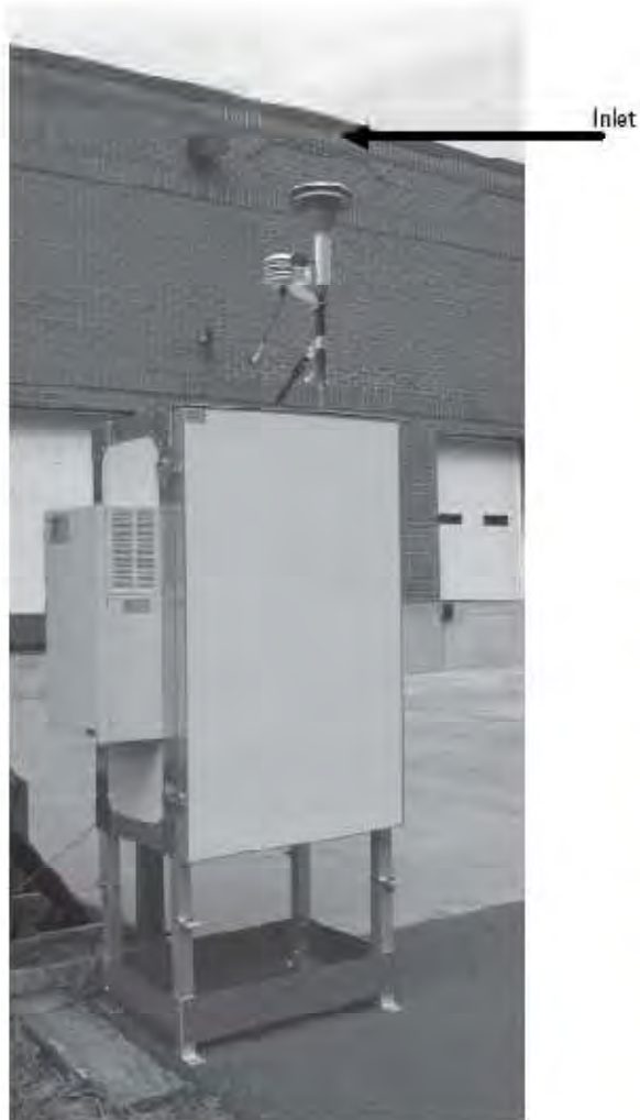
Figure 2-30. Outdoor enclosure with inlet installed.
