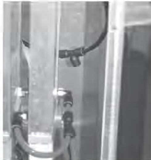
Figure 5-40. Main dryer vacuum line removed from T-fitting.
