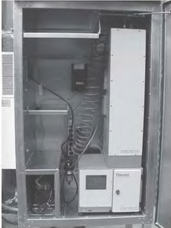
Figure 2-20. 1405 unit in the outdoor enclosure.
