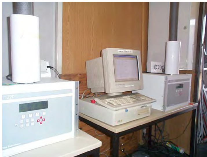
Figure 7: Measuring systems BAM-1020, installed in measurement cabinet
