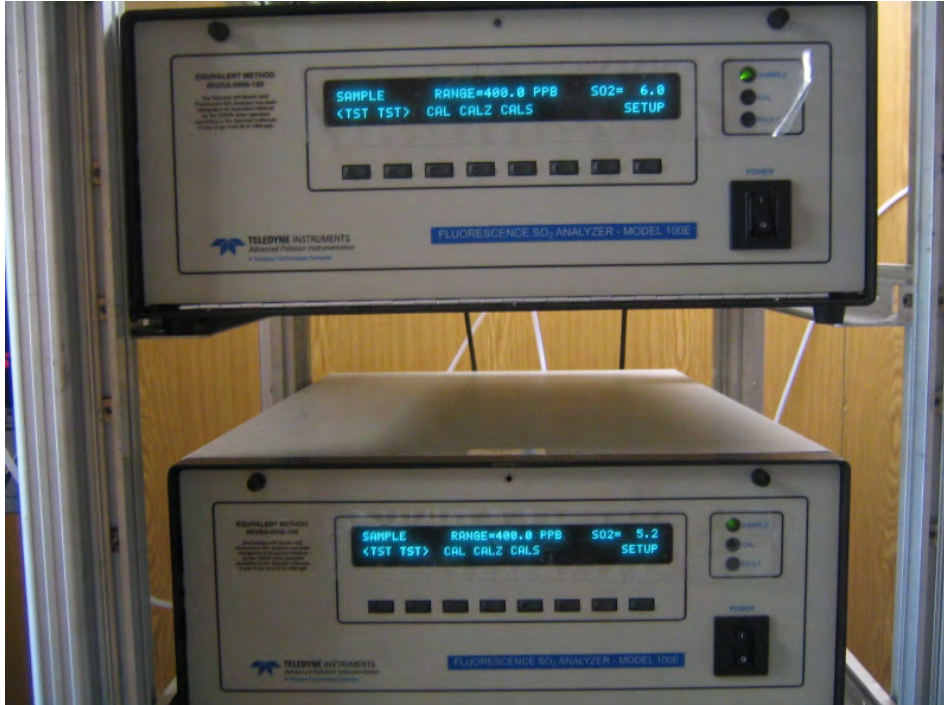
Figure 6: Picture of the analyzers in the measuring container
